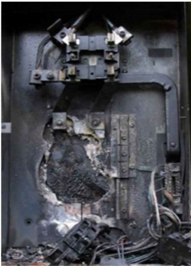
Result of an electrical panel fire.
