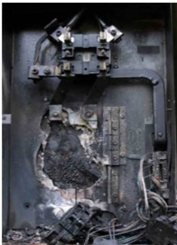
Result of an electrical panel fire.
